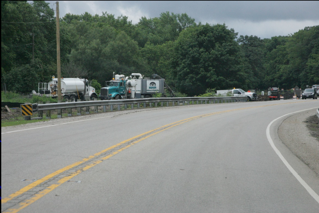
Rain doesn't stop utilities from relocating on the LMP Section B-2 project
