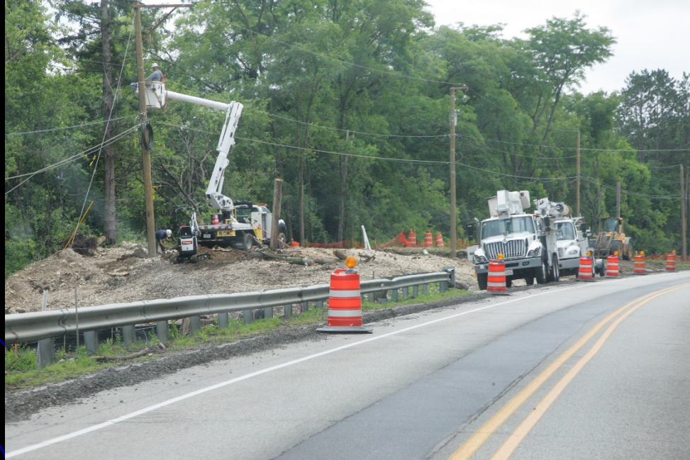
Crews continue utility relocations and storm sewer installation on the LMP Section D - IL 25 to IL 62 project
