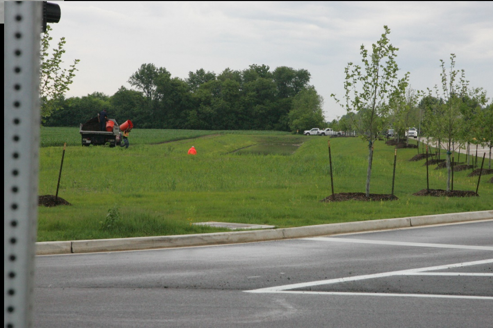
Landscaping crews work on punch list items as the contractor wraps up the LMP Section A-2/B-1 - Randall to Karen Drive project
